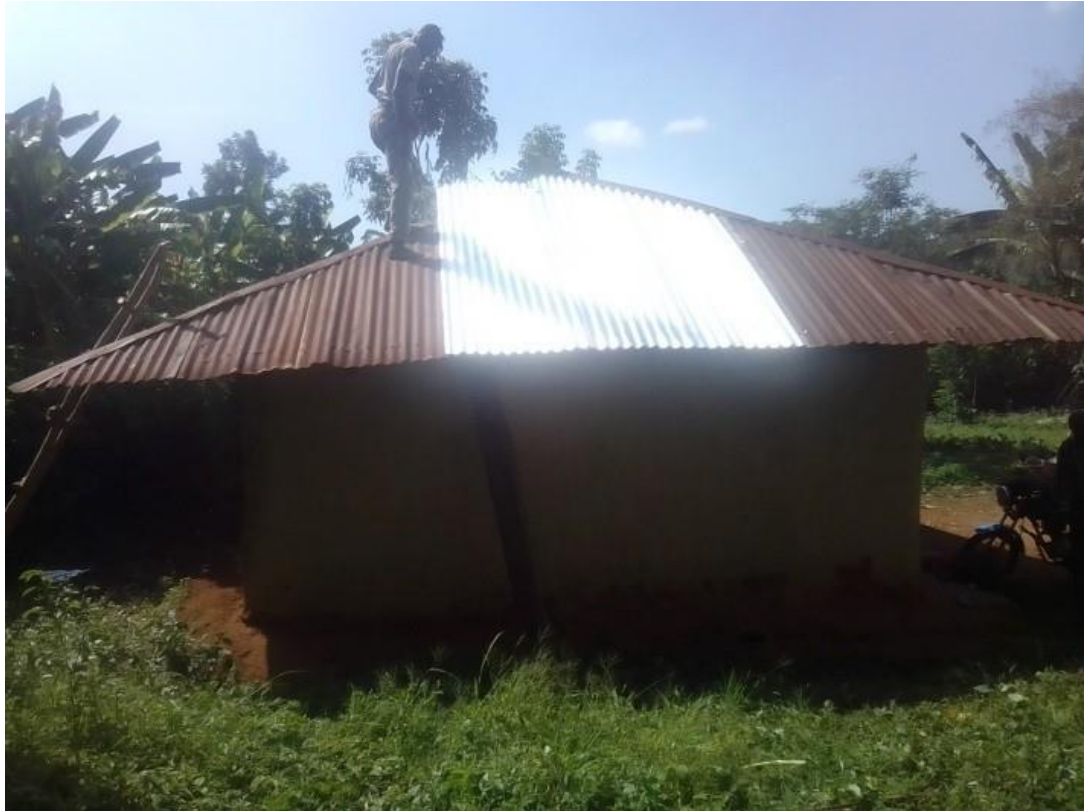
This is one of the two roofs repaired during the last quarter.
