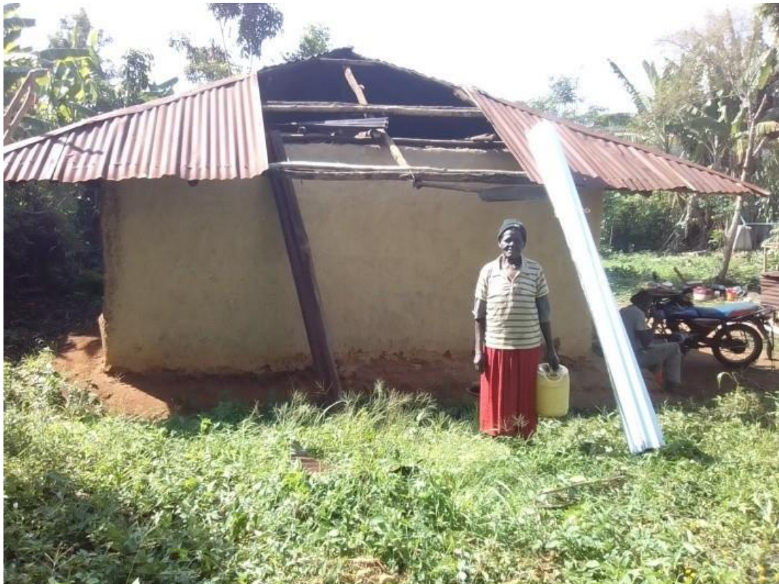
This is one of the widows who benefited from house repair project. Some parts of her house roof had been seriously leaking.
