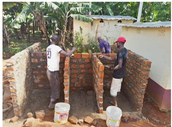
Replacement of Latrines – damaged in recent heavy rains - for use by the Pupils
